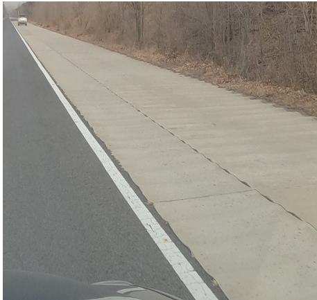
Dislocated Washboard Road C
